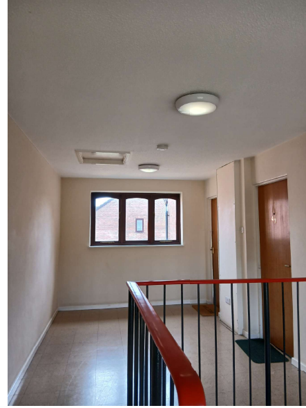
Lighting (Standard and Emergency Lights)
